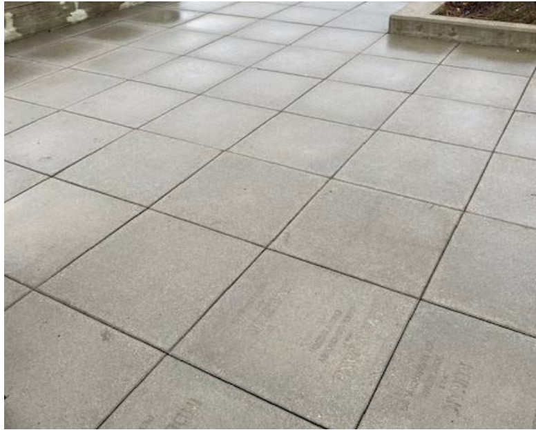
Image 1: Existing Concrete Pavers in Wet Conditions
