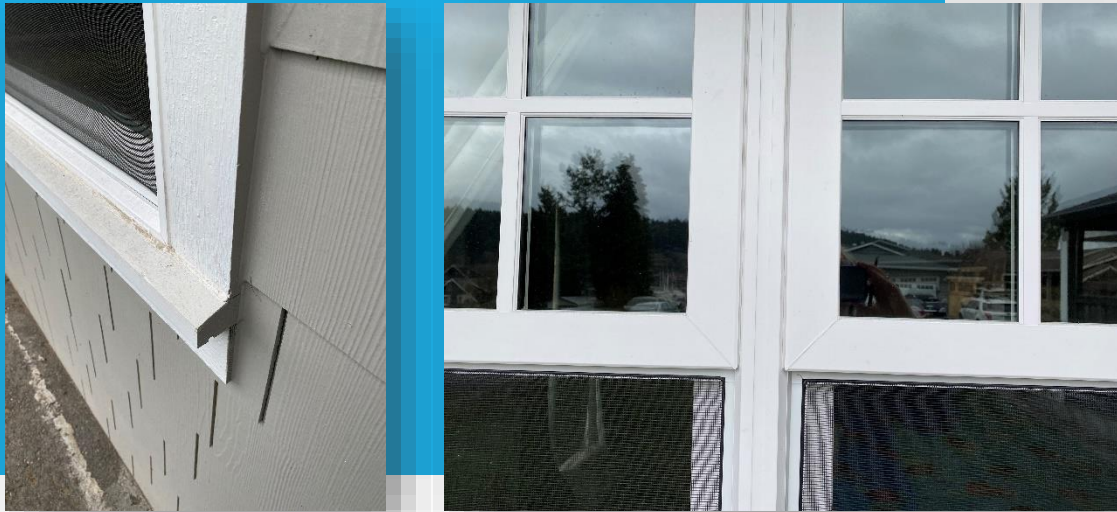
Photos of existing installed grids and trim
