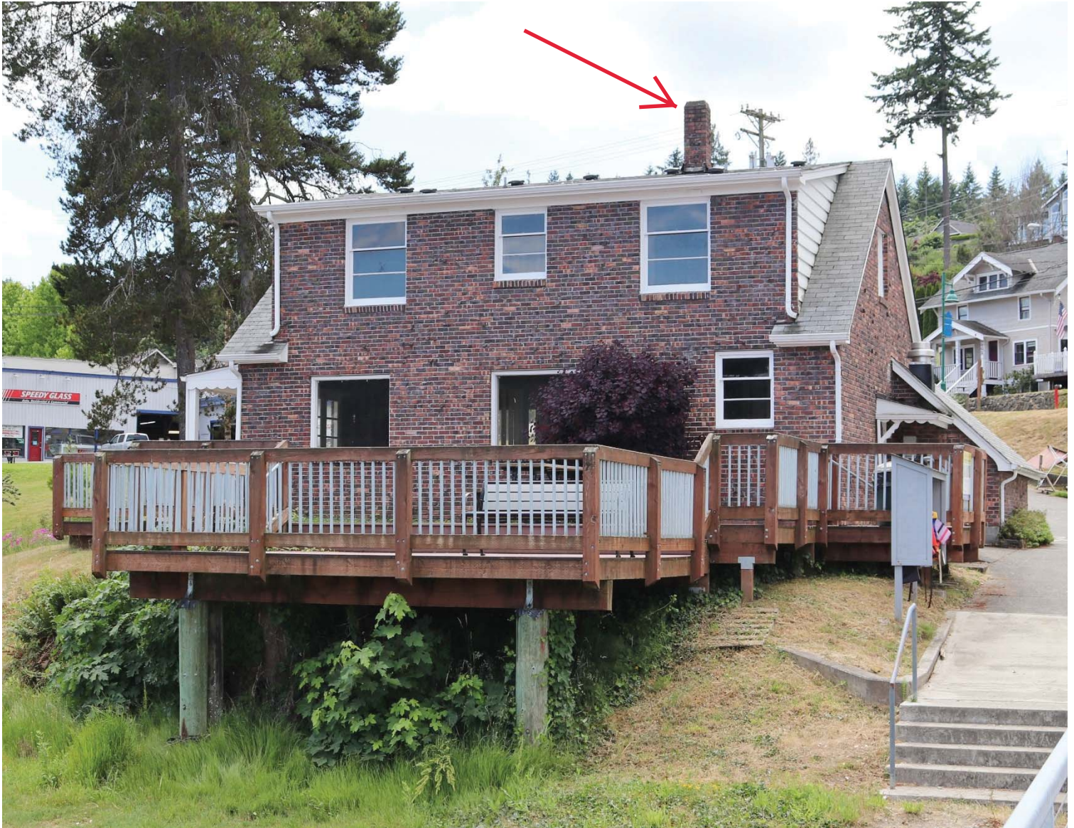
Location of unstable brick chimney – back view
