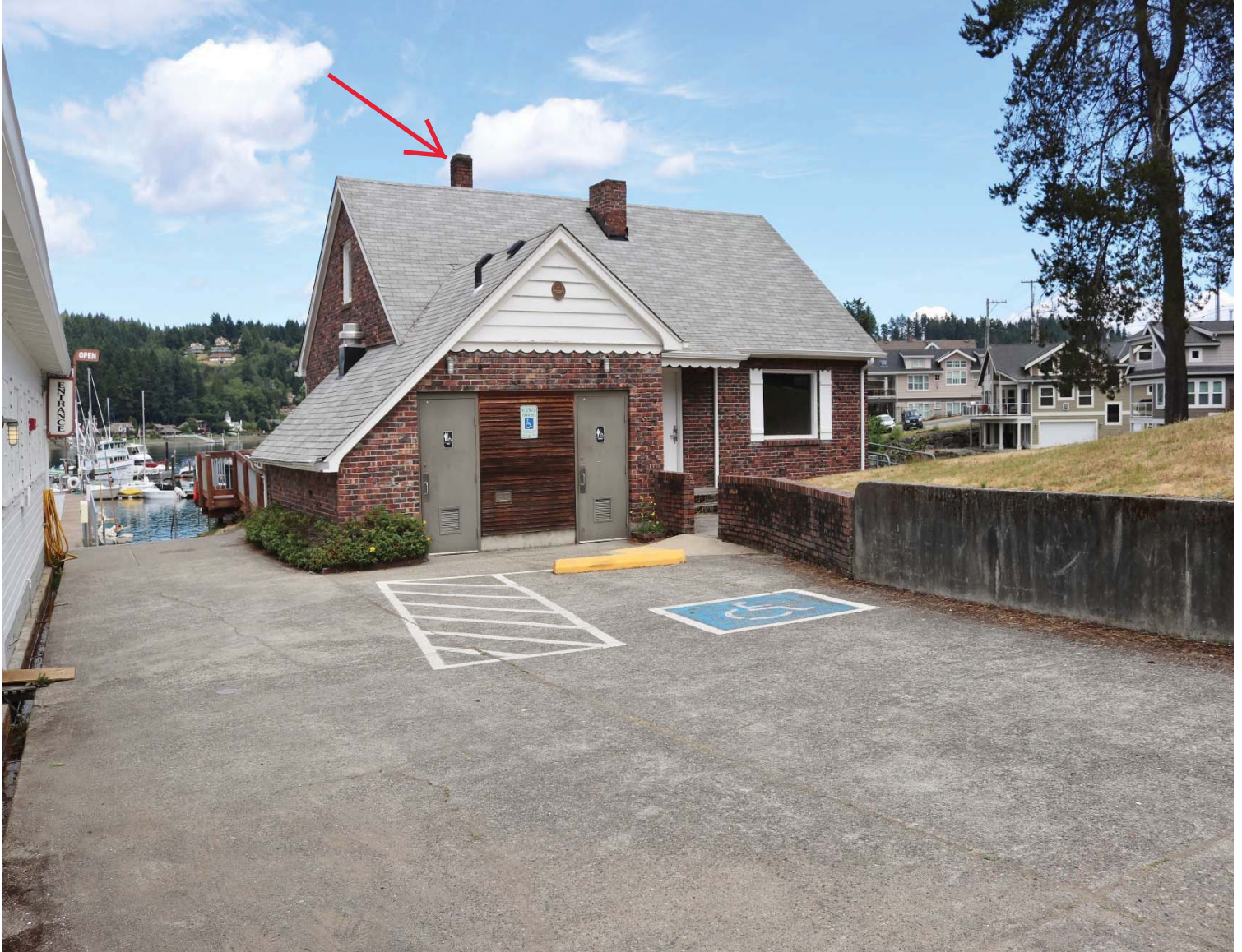
Location of unstable brick chimney – front view
