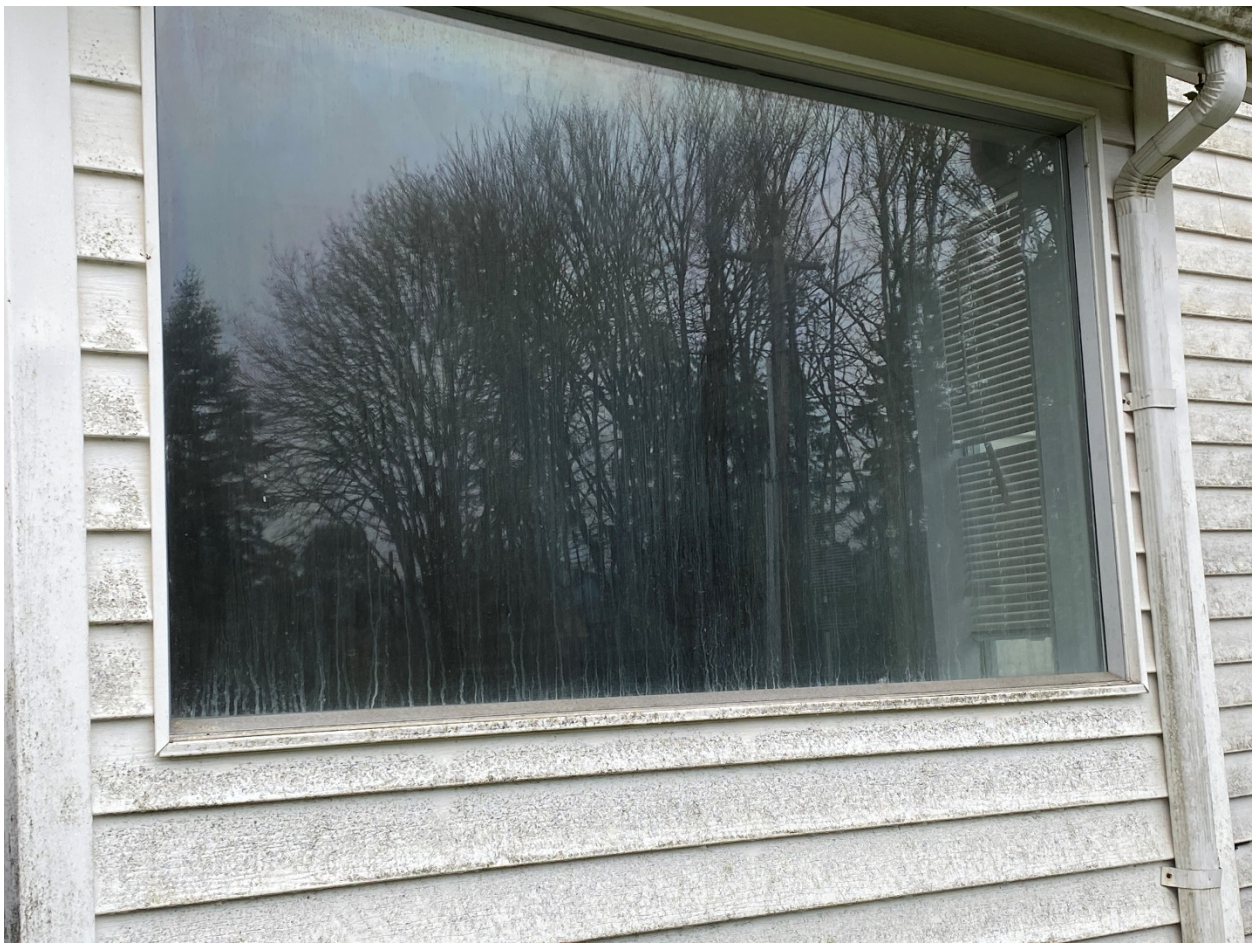
2 Mildewed siding and cloudy picture window
