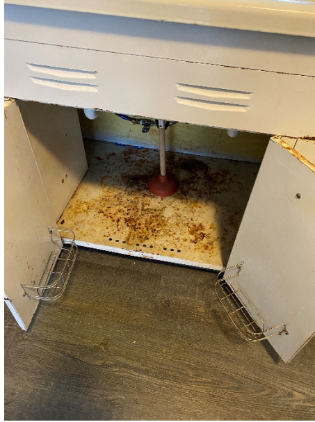
Rusty sink cabinet
