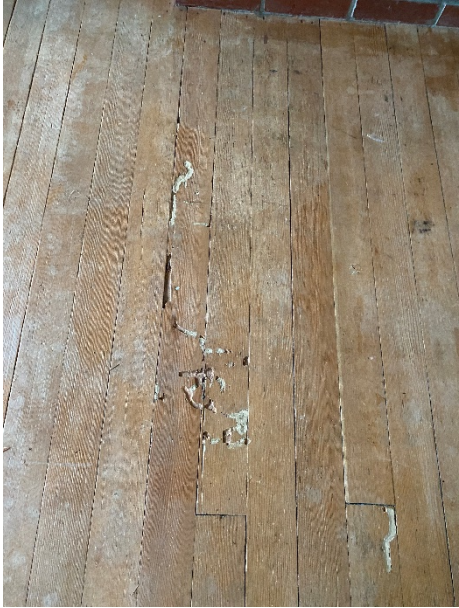
1 Termite damage in floor
