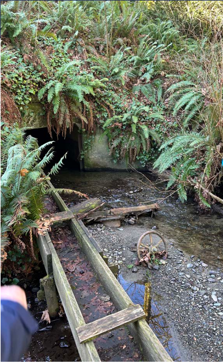
Flow control valve in disrepair - 2025
