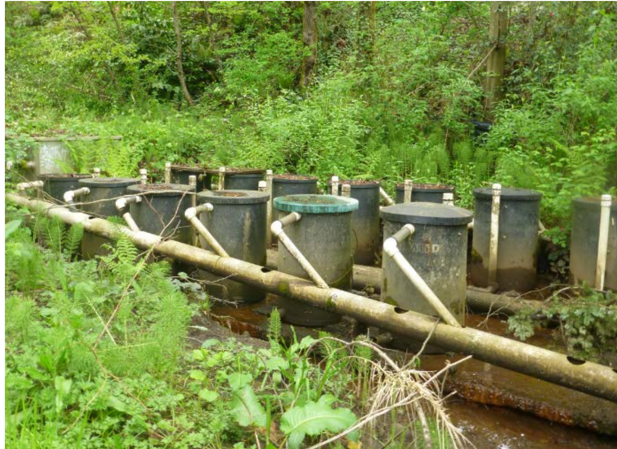
RSIs in disrepair - 2024
