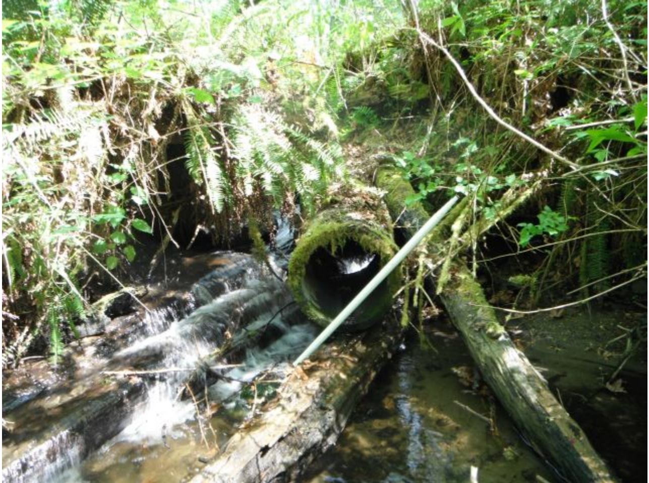
Culvert under former driveway. Driveway and culvert are both washed out and form a partial stream blockage. Photo courtesy WDFW.
