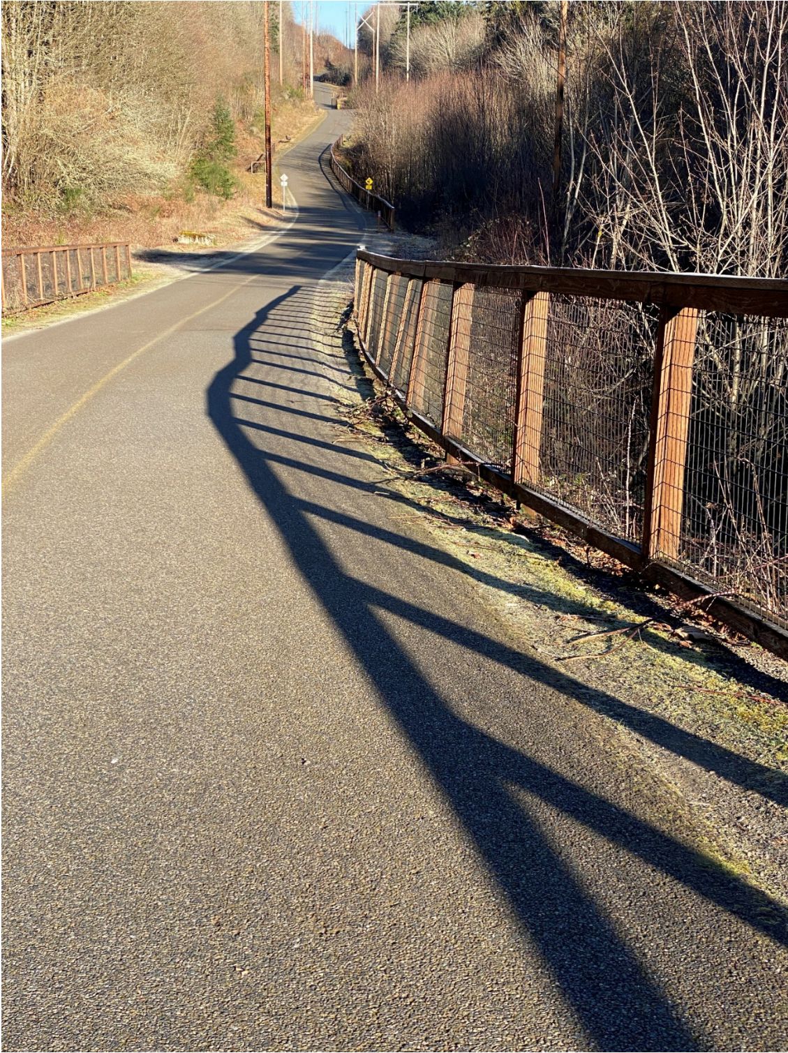
East railing leaning toward ravine
