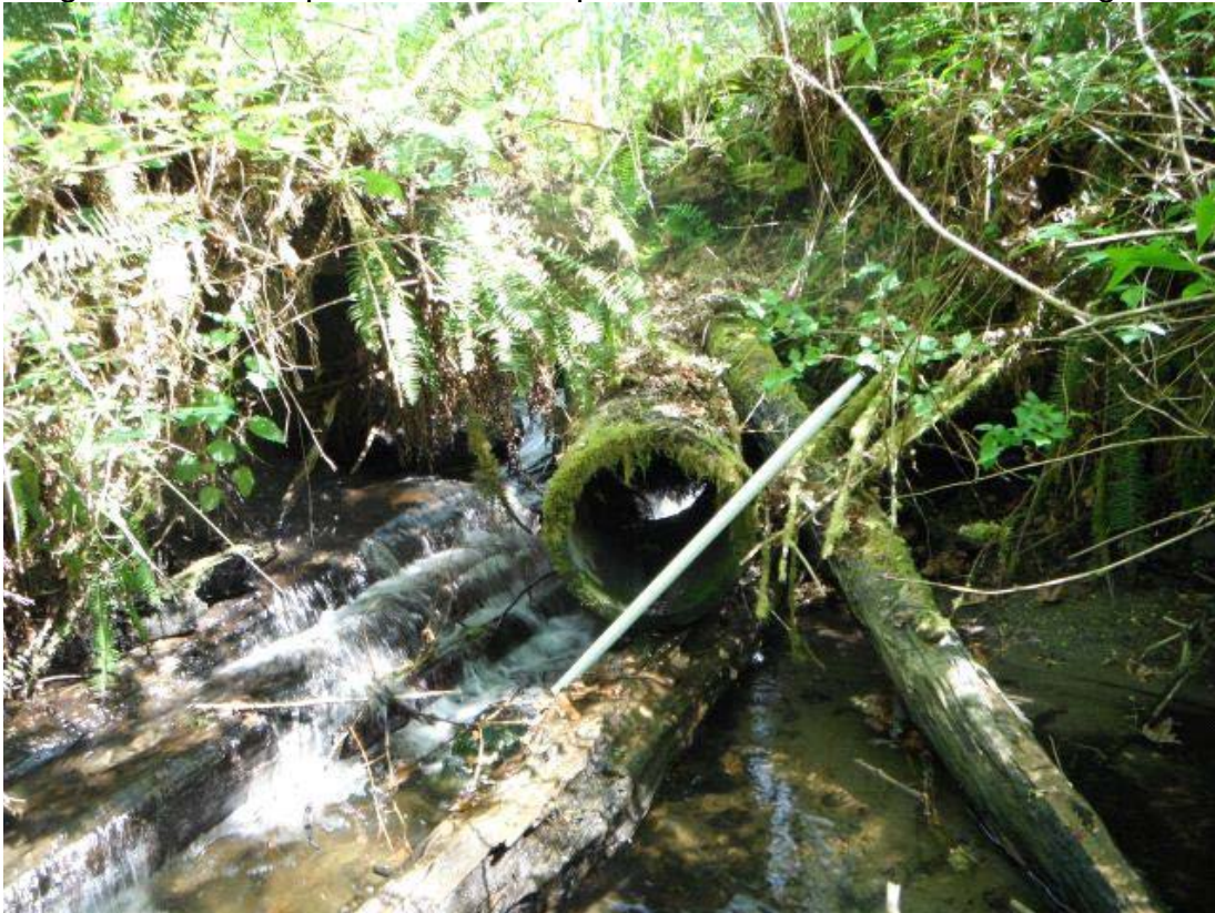
1 Fish & Wildlife photo of driveway washout on Phase 4 property
