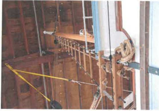
Top left: Below deck the crew quarters are still being pieced back together. Knees (the braces holding up the deck) and stringers (the long boards running horizontally) will remain in view as part of the preservation plan.
